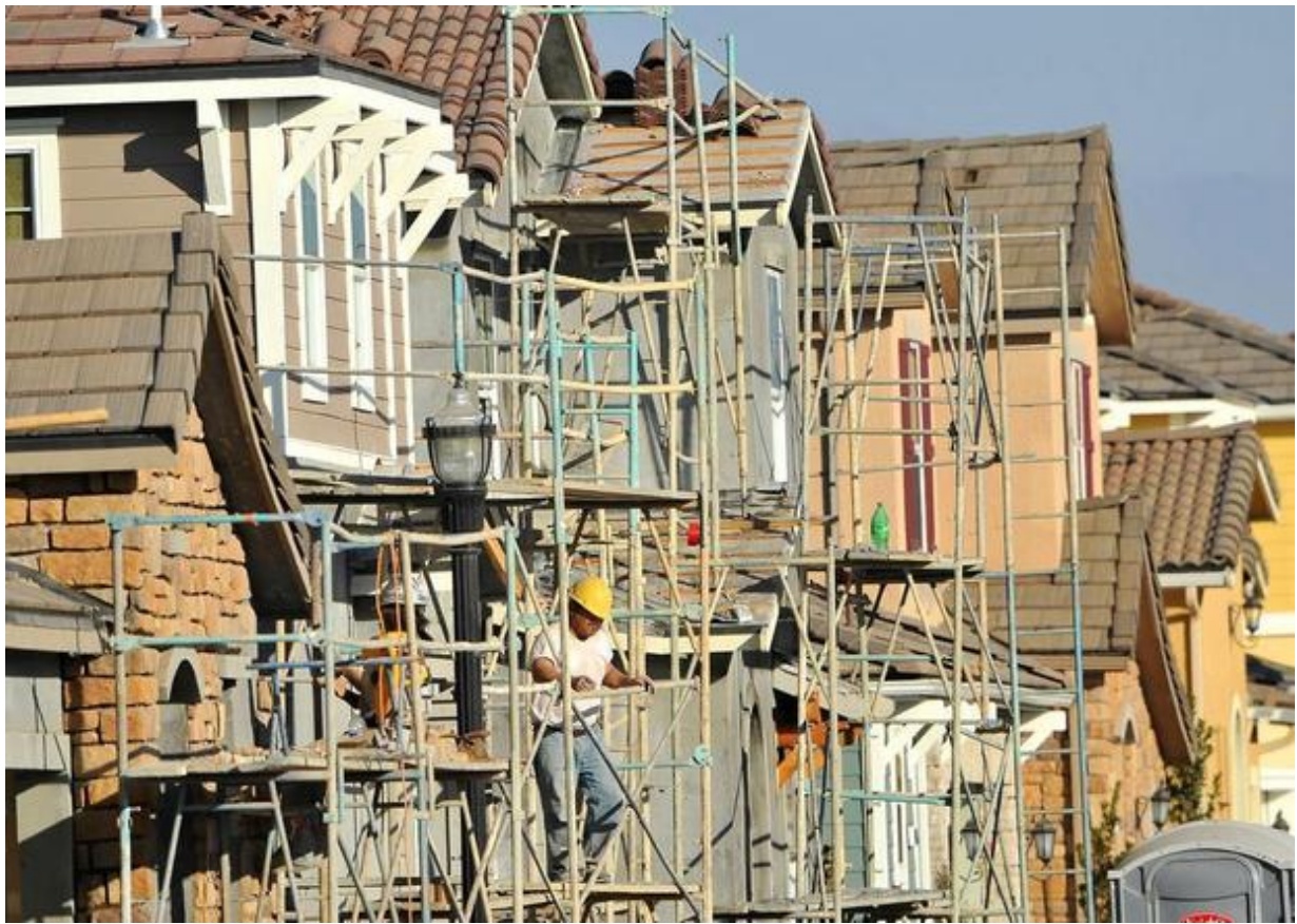
Home construction at Harlan Ranch is seen in a January 2014 file photo. JOHN WALKER — THE FRESNO BEE
