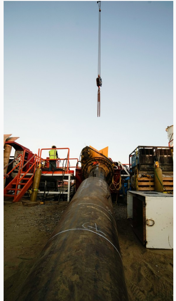
California American is using directional drilling extend a pipe some 735 feet under the beach, in hopes of sucking in a couple thousand gallons of seawater per minute from below the ocean floor. (Luke Gianni/California American Water Co.)
